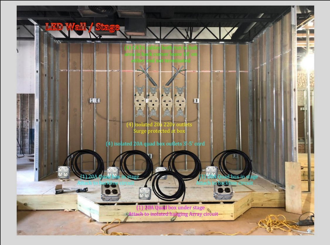
Isolated circuits, surge protection, and CAT6 backbone — wall & VIP display
